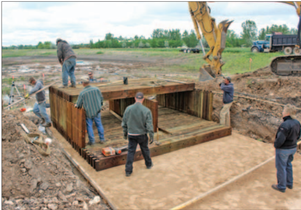
A crew works Wednesday to install a timber box culvert in the Ward Development in the Exit 8 vicinity of Spearfish. Designers said that the culvert will likely last longer than the road that will eventually be built over the culvert. Pioneer photo by Kaija Swisher
